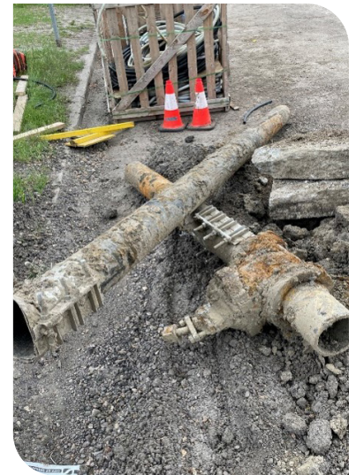
Old Cast Iron Pipe
