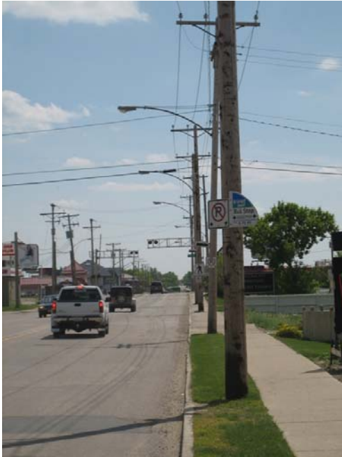
Overhead power lines
