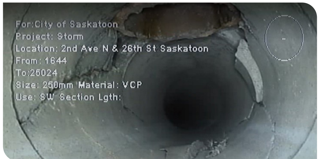
Sewer Pipe Condition Assessment Very Poor
