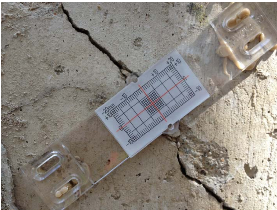
Photo F.5: Crack Meter Located on the West Face of the Retaining Wall Between 230 & 306 Sask. Cres. E. (CM3) (Aug 12, 2013)
