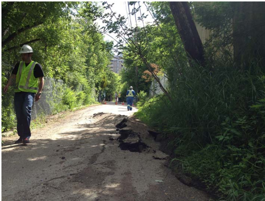
Photo C.6. Bulging Toe of Slide on Cherry Lane (June 21, 2012)
