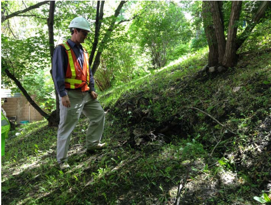
Photo C.7. Bulging Toe of Slide below Cherry Lane (June 21, 2012)
