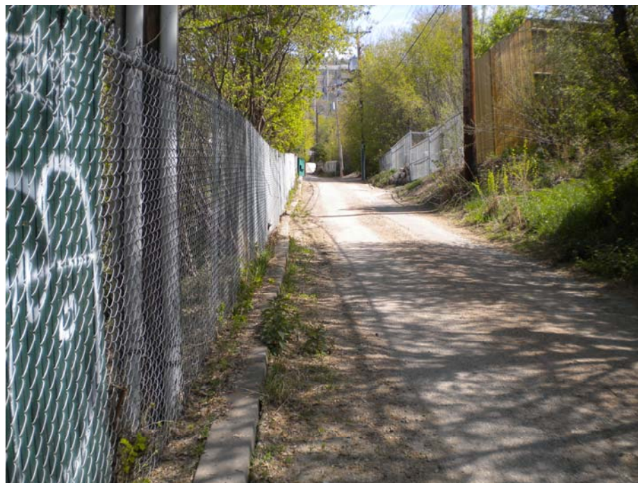
Photo C.2. Looking East at Deflection of Curb and Fence Line along Cherry Lane (May 27, 2010)
