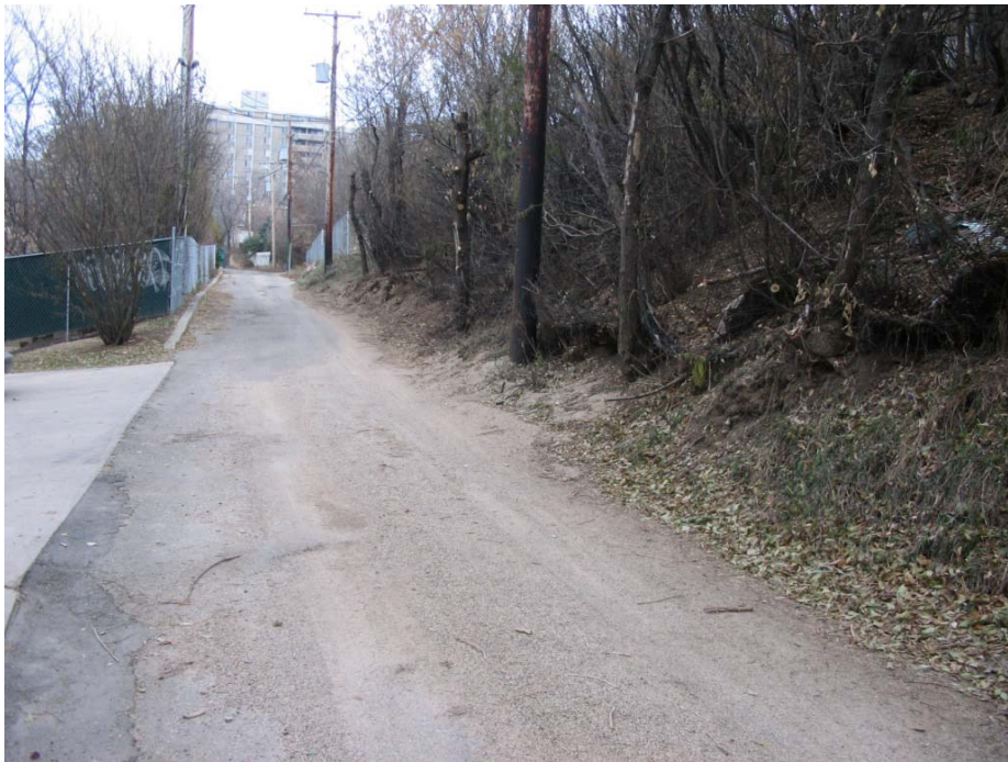
Photo C.1. Looking East at Deflection of Curb and Fence Line along Cherry Lane (Nov 5, 2006)
