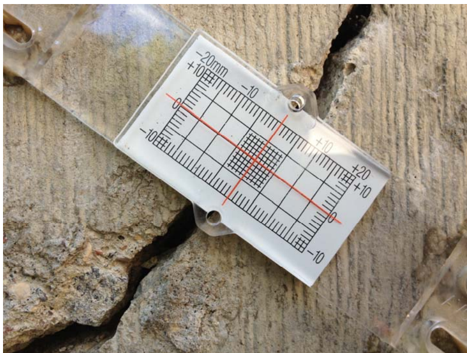
Photo F.3: Crack Meter Located on the East Face of the Retaining Wall Between 230 & 306 Sask. Cres. E. (CM2) (Aug 12, 2013)
