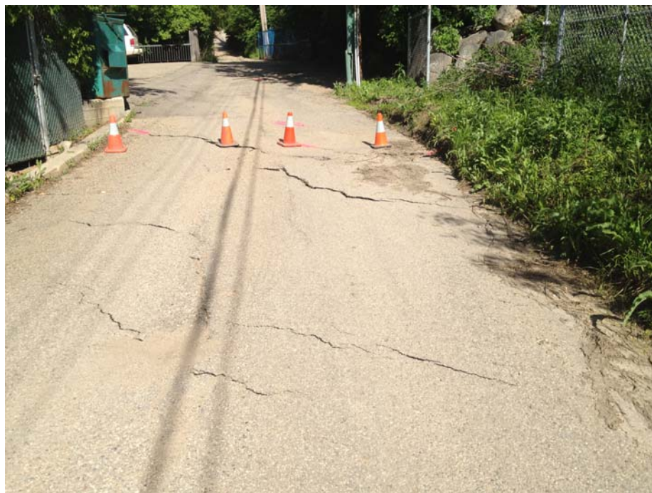
Photo C.10. Looking East at Tension Cracking along Cherry Lane (June 21, 2013)
