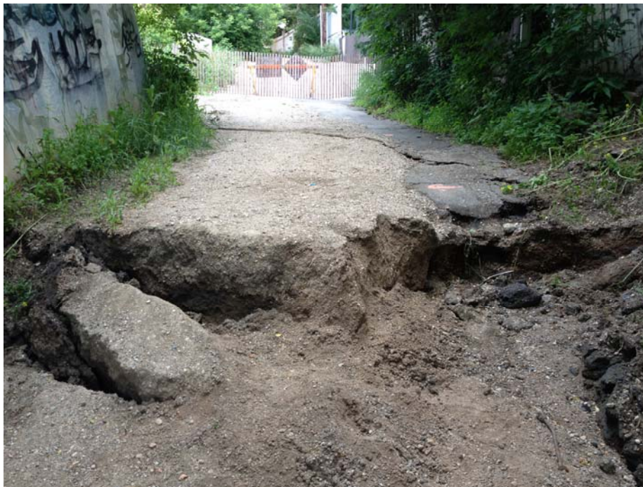
Photo C.20. Looking East at Drop in Pavement behind 305 11th St. E.; Approx 53 cm Drop (June 4, 2013)
