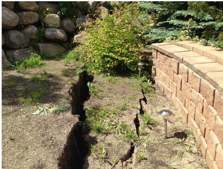
Photo C.8. Cracking Behind Retaining Wall in Backyard of 237-239 11th St. E. (June 21, 2012)
