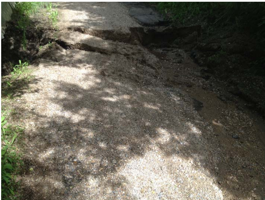
Photo C.15. Looking East at Severe Cracking across Cherry Lane, Pavement; Approx. 50 cm Drop (June 24, 2013)
