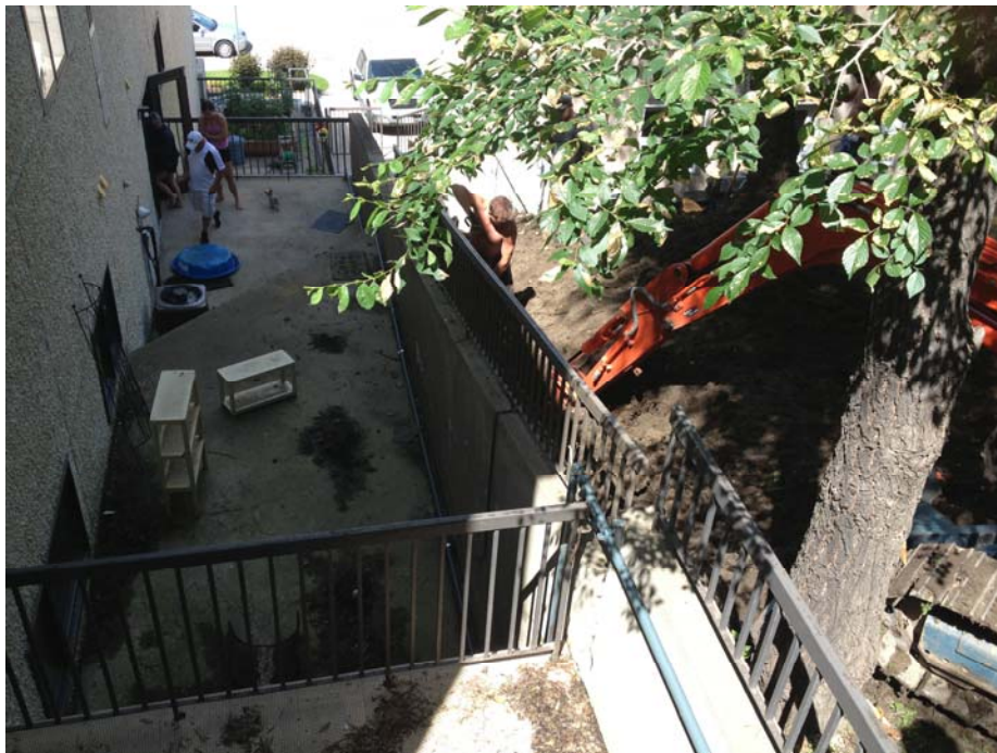
Photo C.24. Looking Northeast at Trench being Excavated Adjacent to Wall between 230 & 306 Sask. Cres. E. (July 7, 2013)
