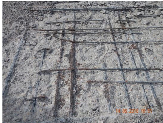
Severe corrosion on the reinforcing steel.
