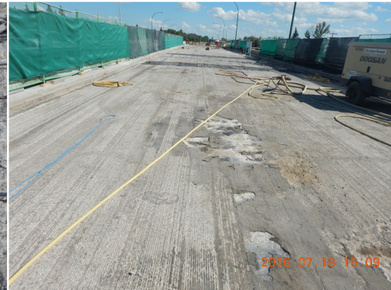
Disintegrated concrete and delaminations that became apparent once asphalt was removed.
