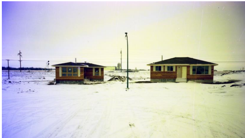
530 and 526 Appleby Place in February 1977, under construction (credit: Photograph CP-7393-B by Creative Professional Photographers courtesy Saskatoon Public Library – Local History Room)
