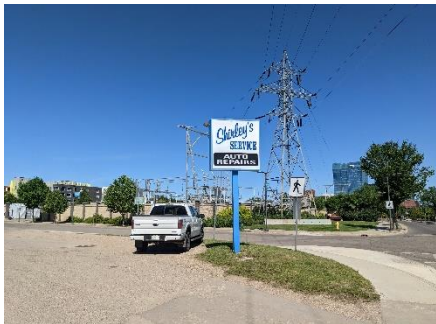
Electrical substation on Avenue C South
