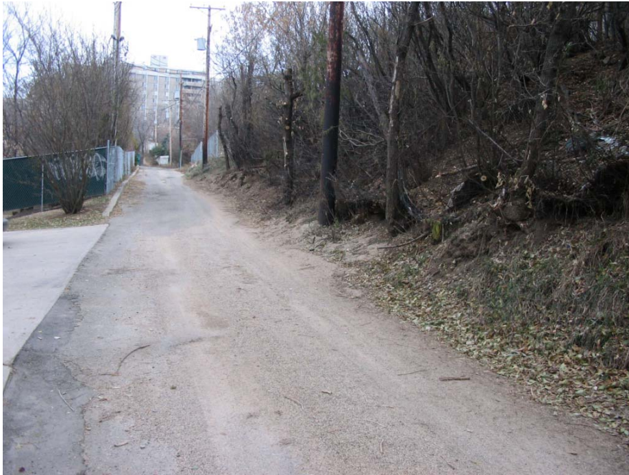
Photo C.1. Looking East at Deflection of Curb and Fence Line along Cherry Lane (Nov 5, 2006)
