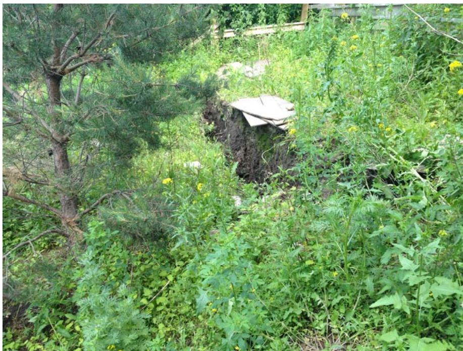
Photo C.12. Looking East at Headscarp of East Failure in Backyard of 305 11th St. E.; Approx. 90 cm Drop (June 24, 2013)
