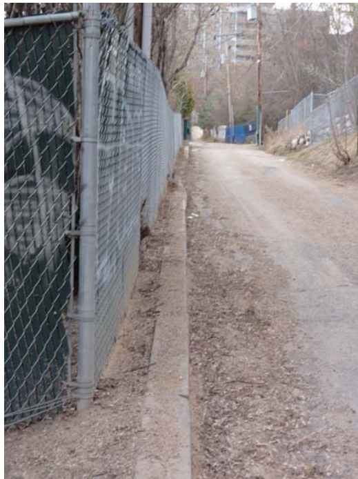
Photo C.3. Looking East at Deflection of Curb and Fence Line along Cherry Lane (April 26, 2012)
