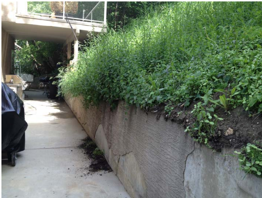
Photo C.14. Looking East at Bulging Toe of Slide above Retaining Wall behind 306 Sask. Cres. E. (June 24, 2013)
