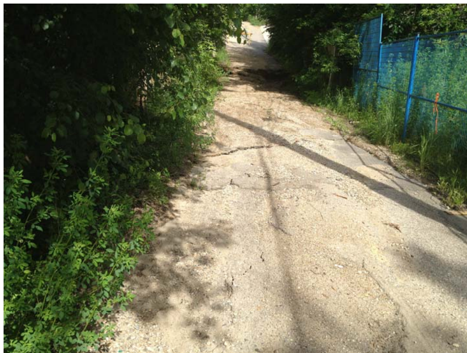
Photo C.16. Looking East at Scarp & Tension Cracking on Cherry Lane (June 24, 2013)
