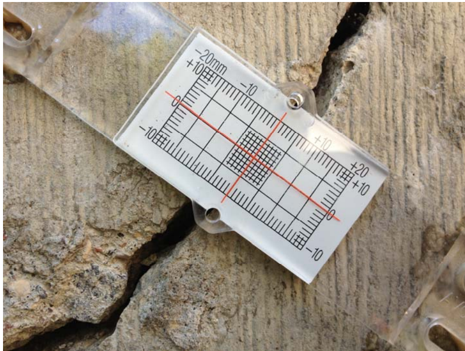
Photo F.3: Crack Meter Located on the East Face of the Retaining Wall Between 230 & 306 Sask. Cres. E. (CM2) (Aug 12, 2013)
