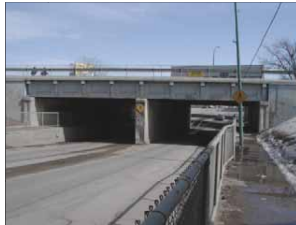
Poor connection - former rail bridge over 19 th Street.
