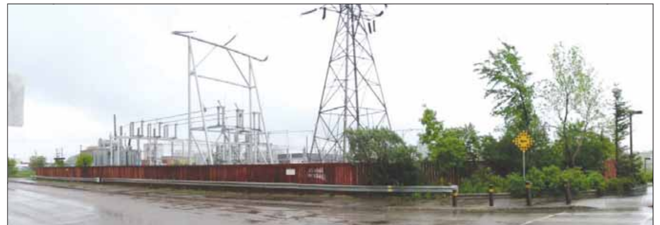
The electrical substation needs a noise wall and landscaping.
