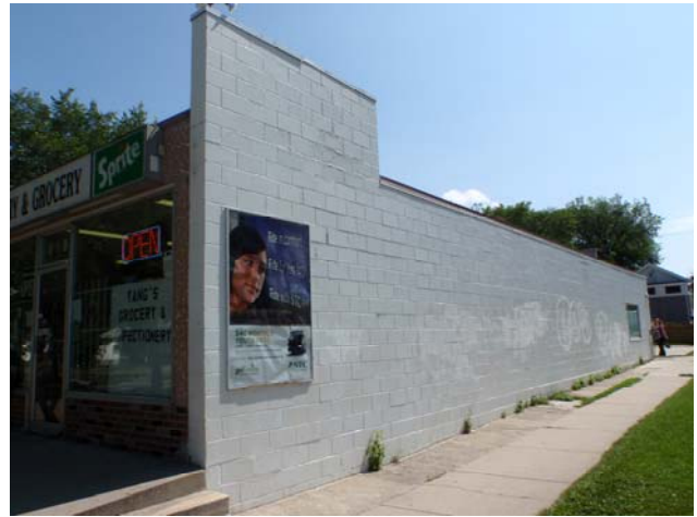
Evidence of graffiti vandalism removed from 29 th Street West convenience store wall
