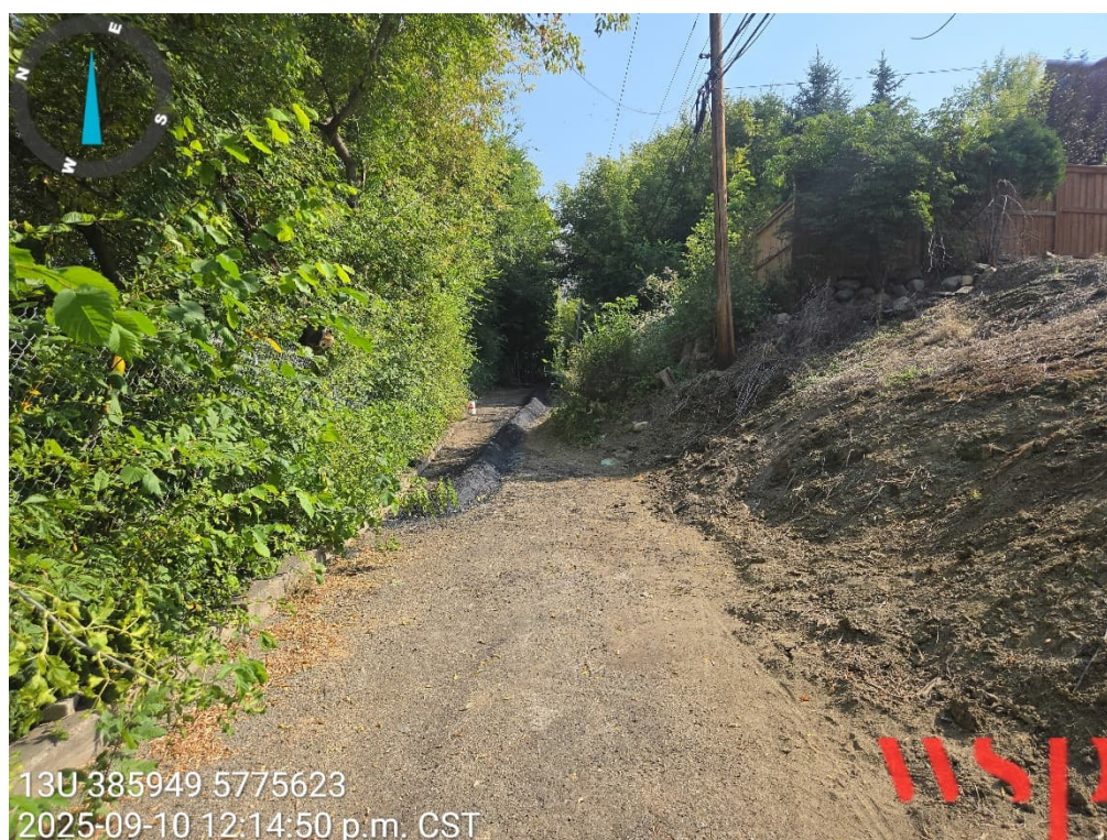
Photograph 2: Looking east down the back alley at the West Failure (September 10, 2025)
