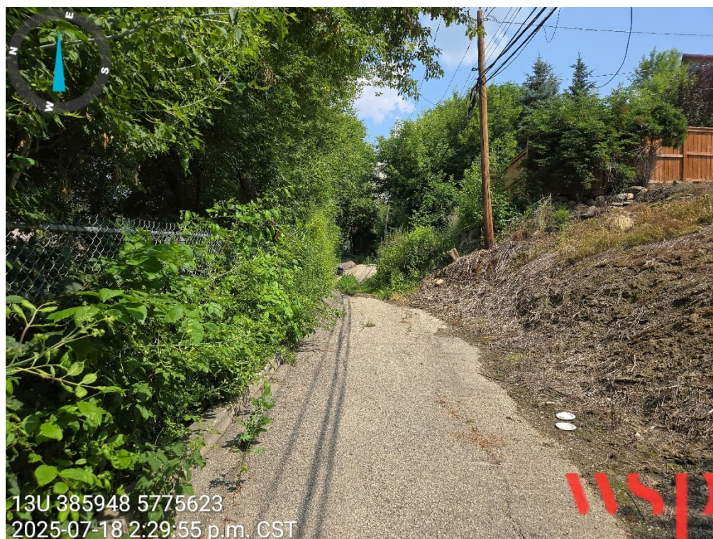
Photograph 2: Looking east down the back alley at the West Failure (July 18, 2025)
