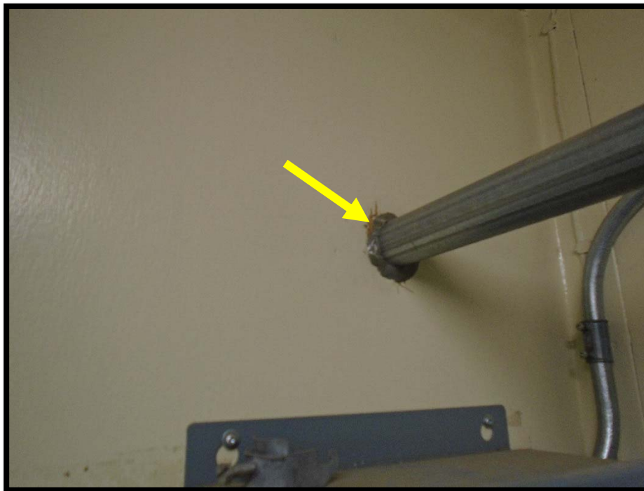
Photograph 1: Asbestos-Containing Grey Firestop Putty.
