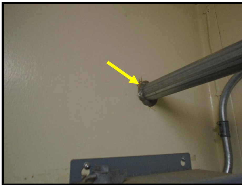
Photograph 1: Asbestos-Containing Grey Firestop Putty.
