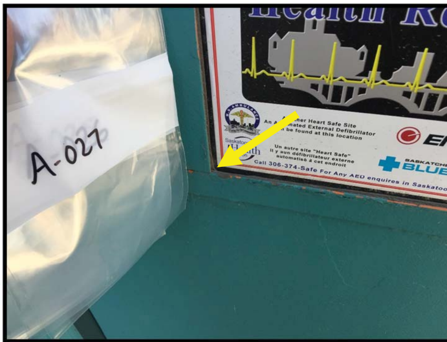
Photograph 1: Asbestos-Containing Black Door Window Caulking.
