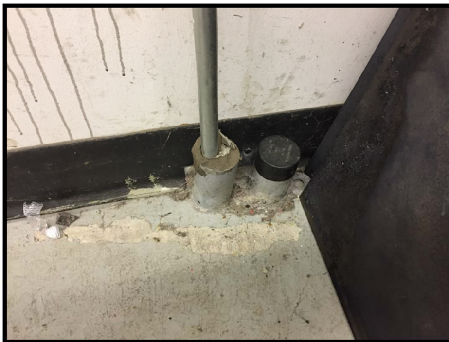
Photograph 1: Asbestos-Containing Grey Firestop.
