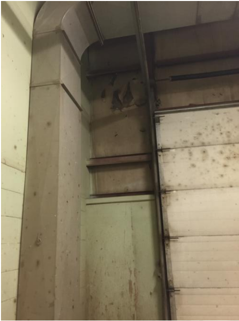
Damaged Wall Insulation
