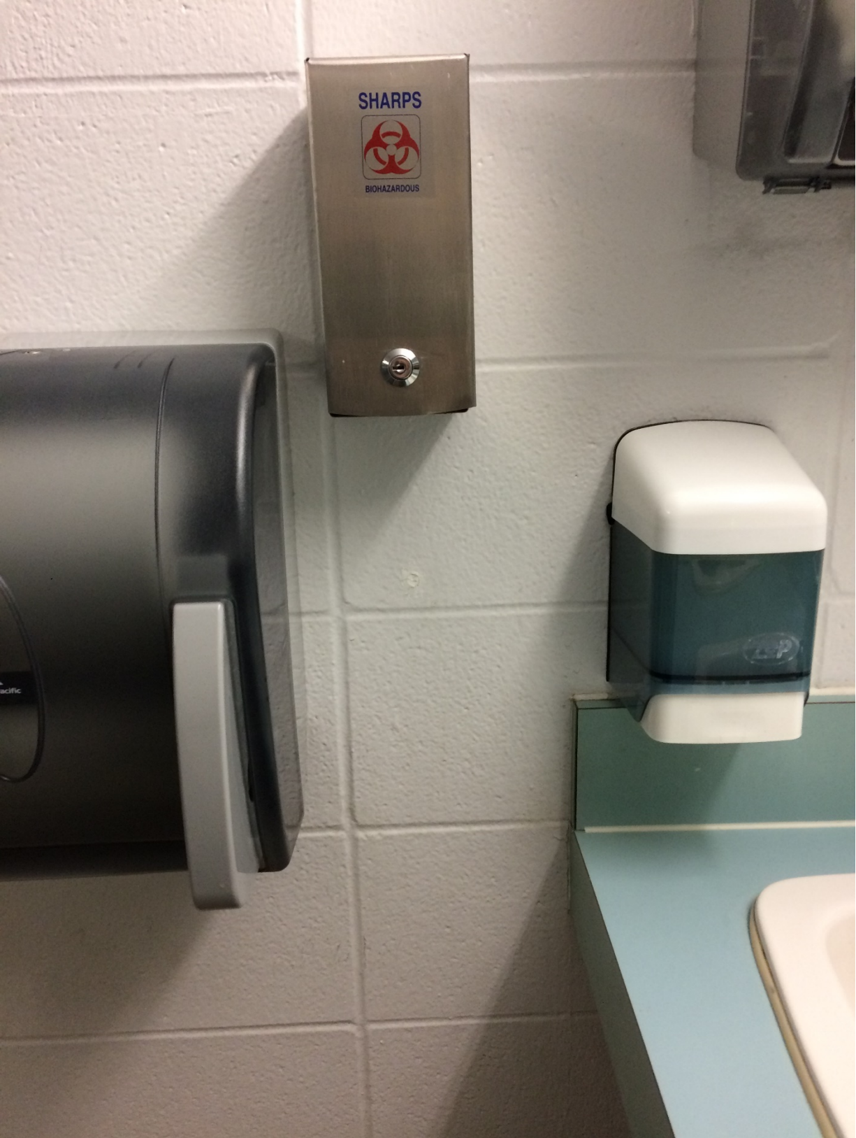
Photo 3- Rm. 145 women's washroom
