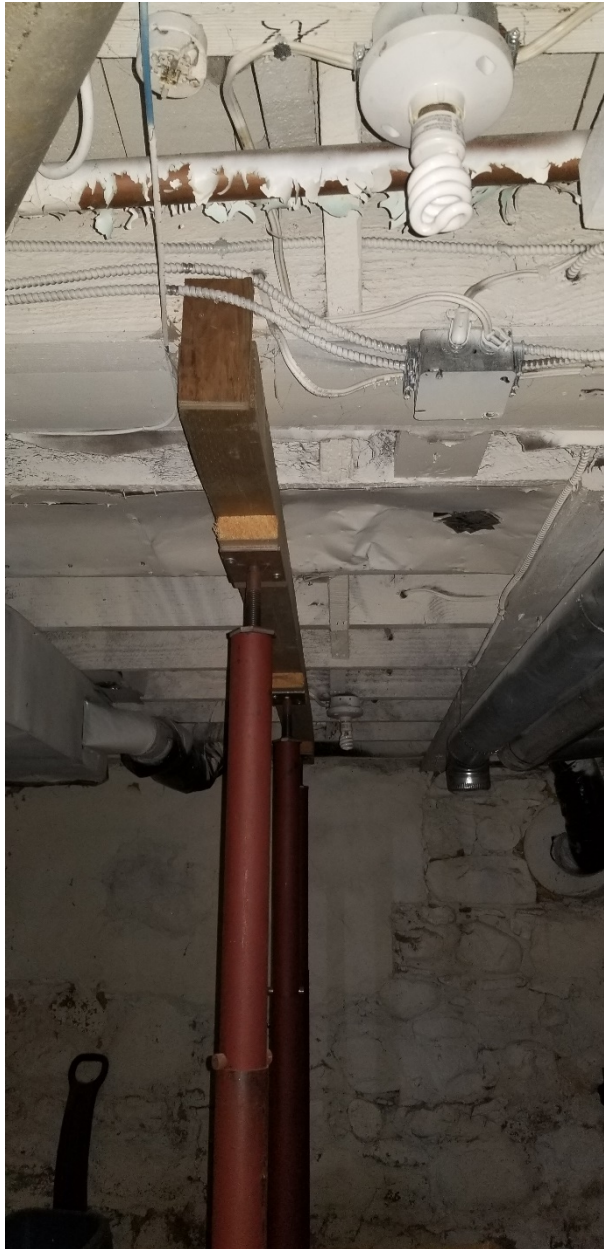
Photo 003- The basement below the main floor living room. No insulation or asbestos containing materials were identified within the truss spaces.
