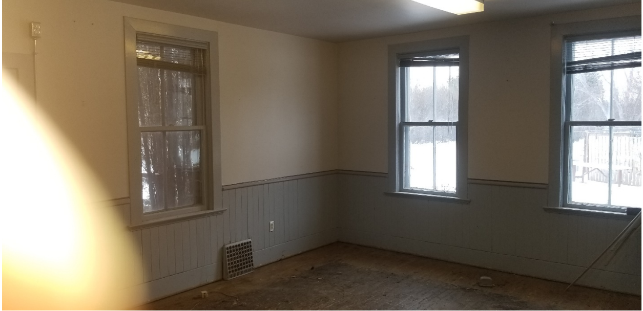
Photo 001- The main floor living room, investigated for the relocation of electrical sockets.
