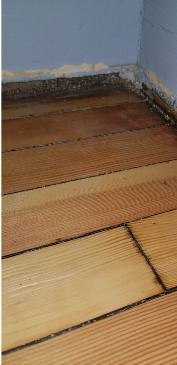
Photo 006- Vermiculite draining from wall in upstairs bedroom.
