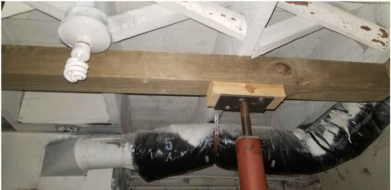
Photo 002- The basement below the main floor living room. No insulation or asbestos containing materials were identified within the truss spaces.
