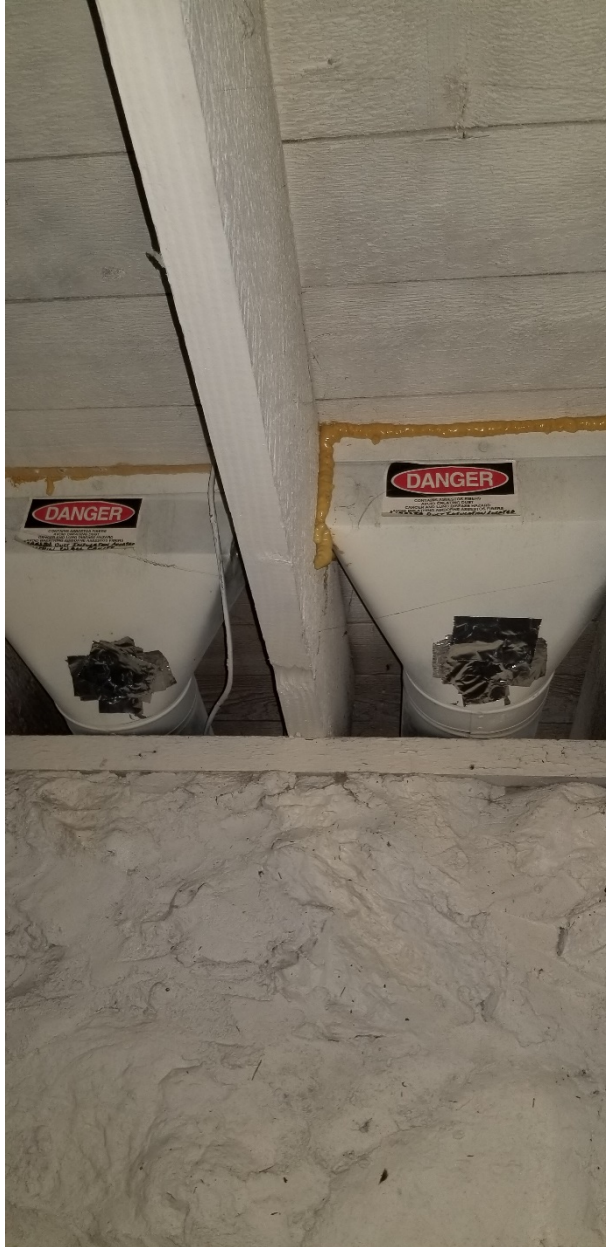
Photo 004- The basement below the main floor living room. Asbestos labels refer to asbestos duct wrap within the wall cavity above the floor.
