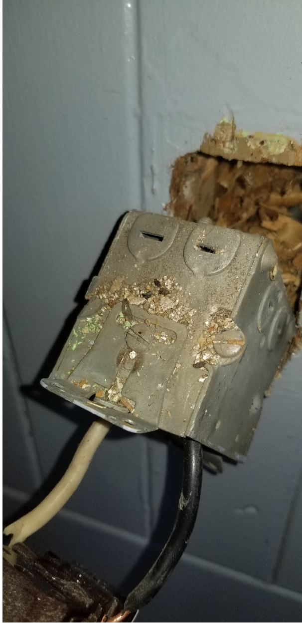
Photo 005- Trace amounts of vermiculite in wall insulation.
