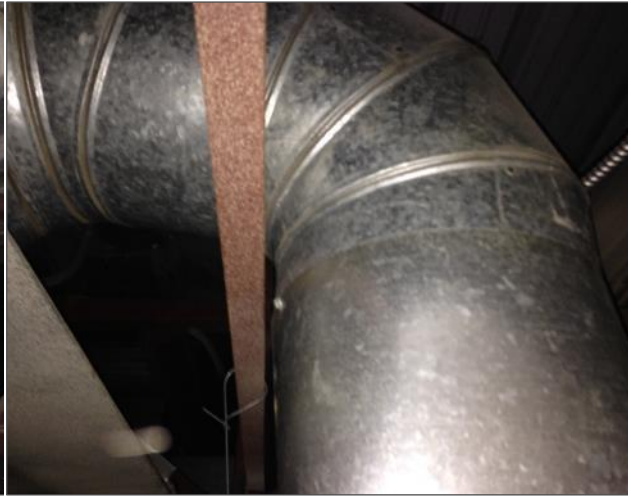
Photo 2: Un-insulated metal duct with no mastic above acoustic ceiling tiles in Men's Washroom (Location 105).
