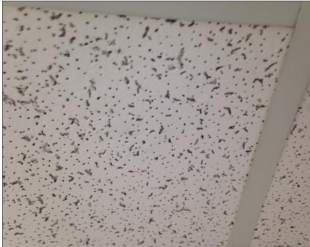
Photo 5: Acoustic Ceiling Tiles, 24"x48" Pinhole and Fissure (Non-asbestos containing Date Stamp 02/08/16), Men's Washroom (Location 105)
