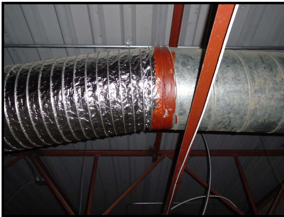
Photograph 2: Asbestos-Containing Red/Brown Duct Mastic.
