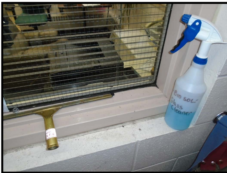
Photograph 1: Asbestos-Containing Black Window Caulking.
