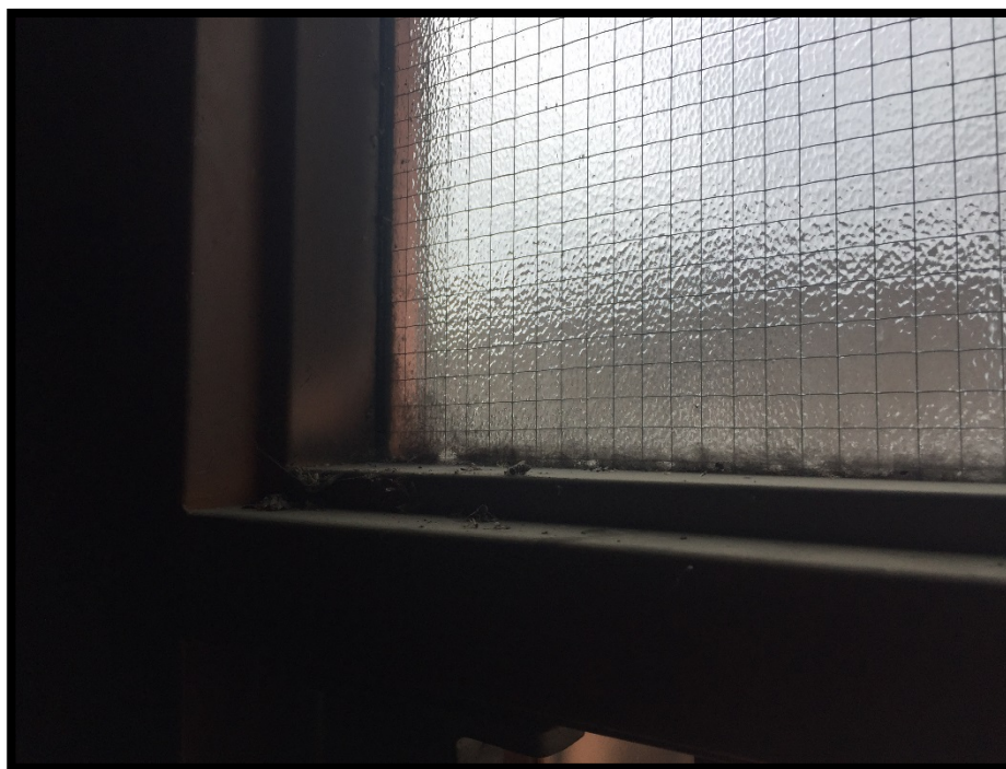
Photograph 1: Asbestos-Containing Black Window Caulking.
