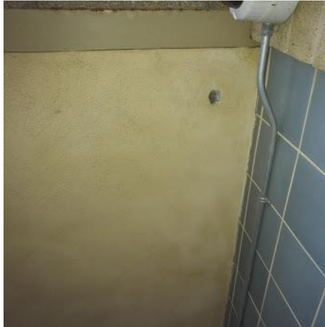
Photo 1: Underside of Main Entrance Overhang Plaster
