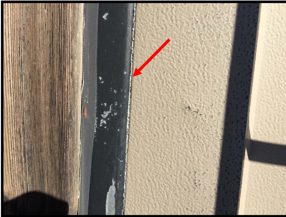
Photograph 2: Asbestos-Containing White Overhead Door Caulking.
