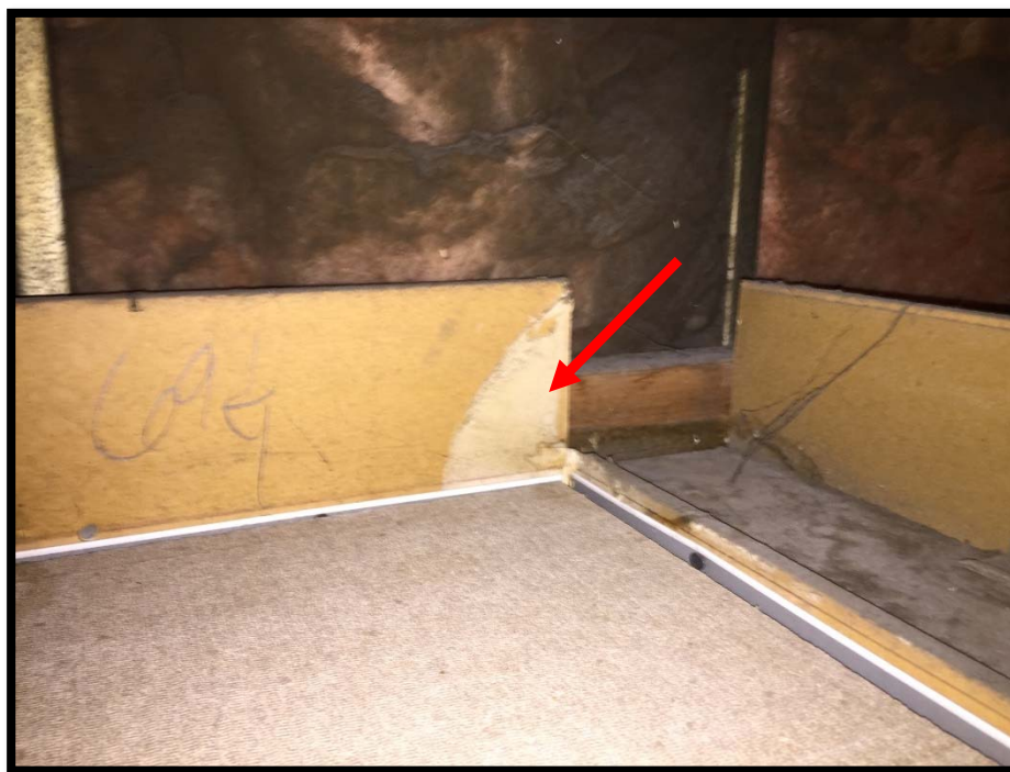
Photograph 3: Asbestos-Containing Drywall Joint Compound.
