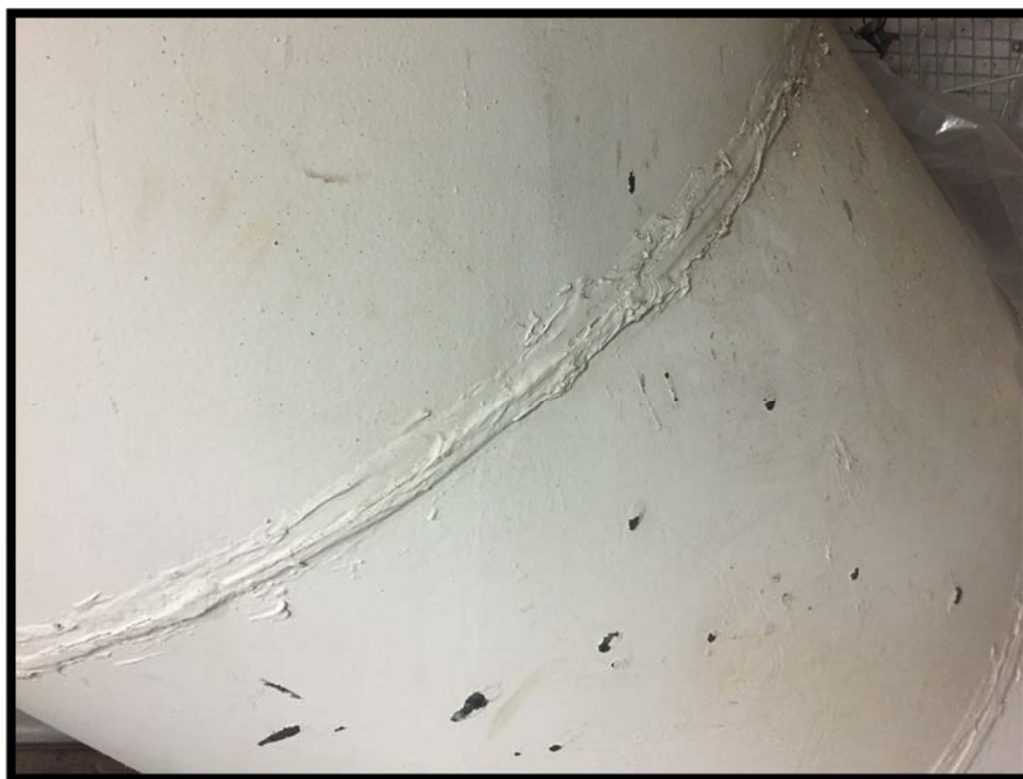
Photograph 1: Asbestos-Containing Tan Duct Mastic (Painted White).
