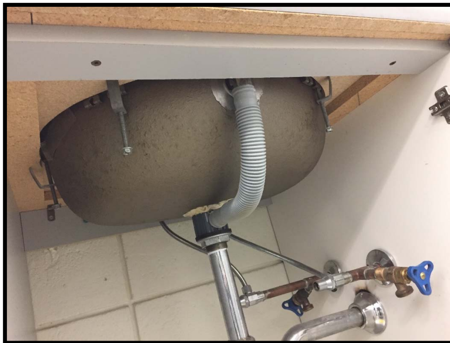
Photograph 2: Asbestos-Containing Gold Sink Undercoat.
