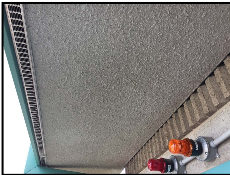
Photograph 1: Asbestos-Containing Concrete Texture Coat.
