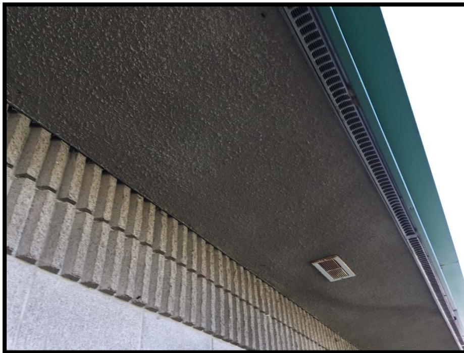
Photograph 1: Asbestos-Containing Concrete Texture Coat.
