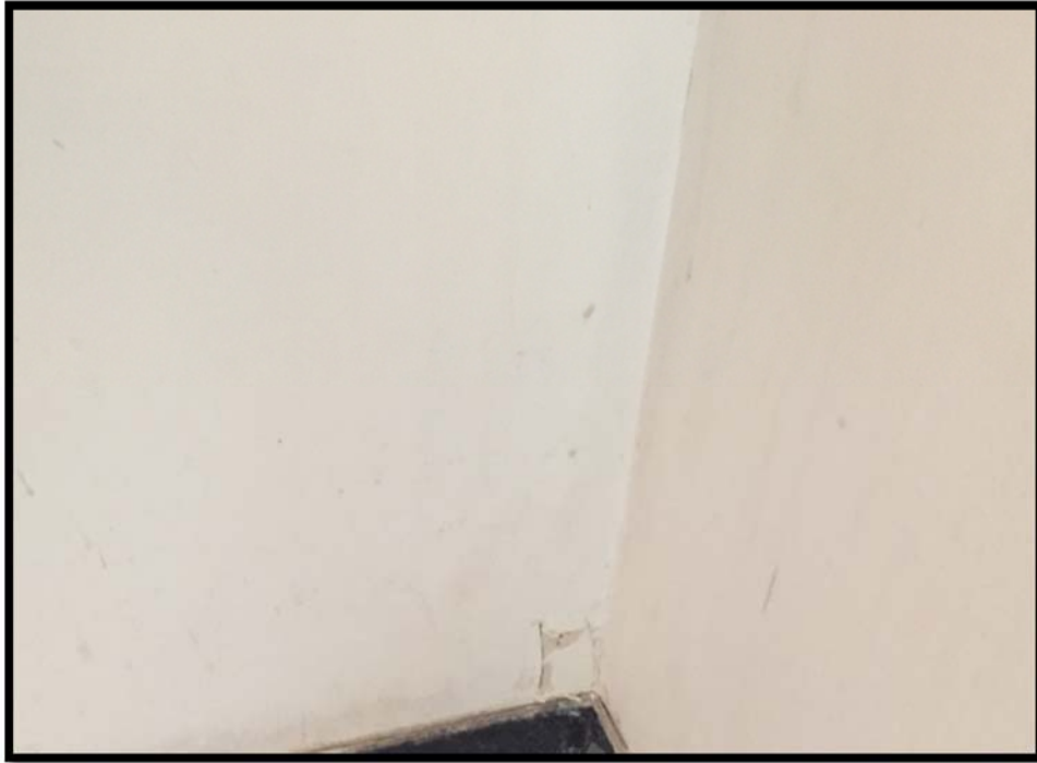
Photograph 1: Asbestos-Containing Drywall Joint Compound.
