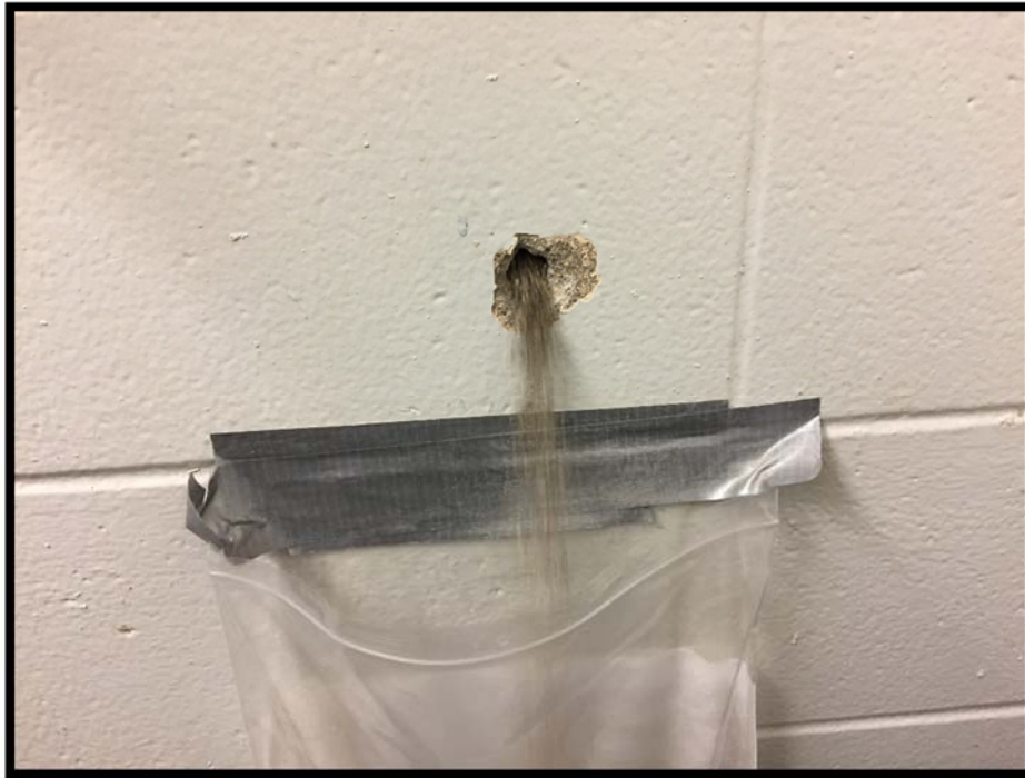
Photograph 2: Asbestos-Containing Vermiculite Insulation.
