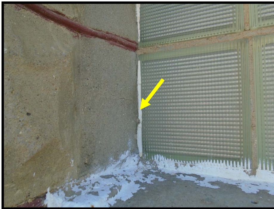
Photograph 5: Asbestos-Containing Exterior White Caulking on Cube Windows
