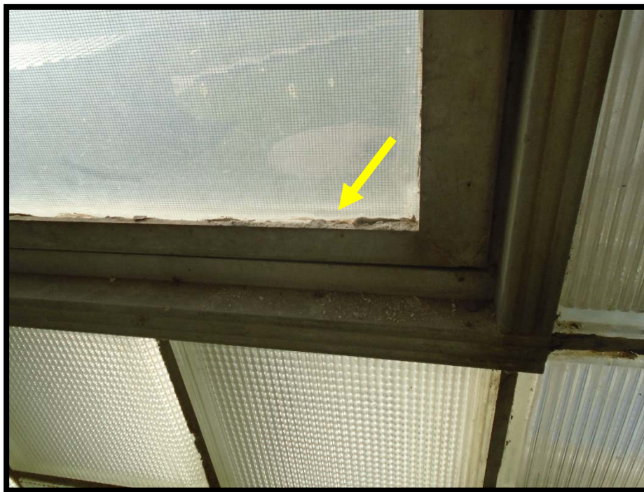
Photograph 2: Asbestos-Containing Grey Window Glazing Below White Caulking.
