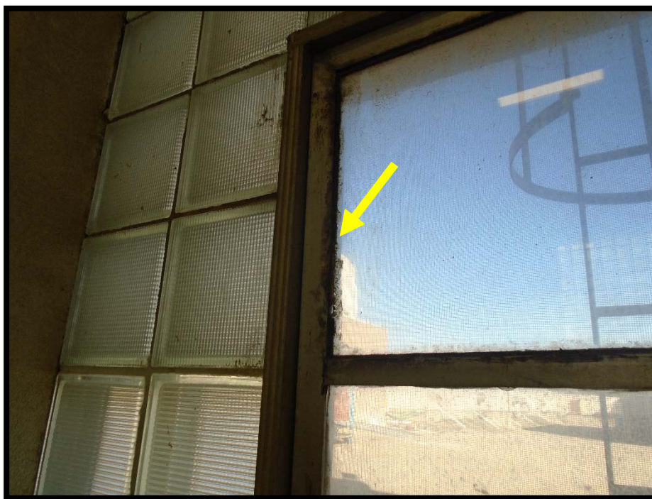
Photograph 1: Asbestos-Containing Black Window Glazing.
