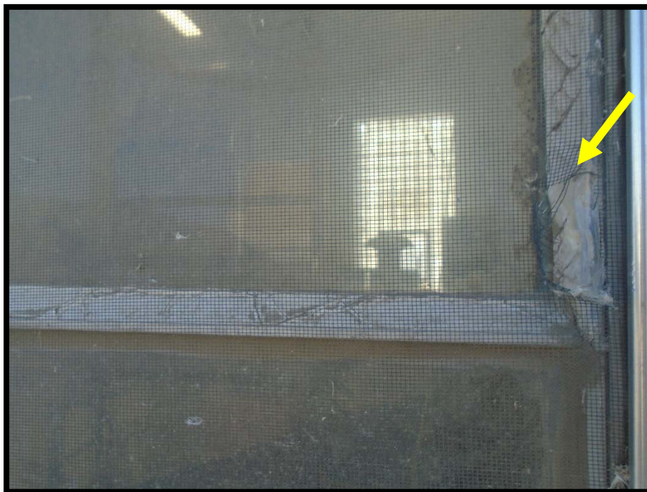
Photograph 4: Asbestos-Containing Exterior White Caulking on Window Pane
