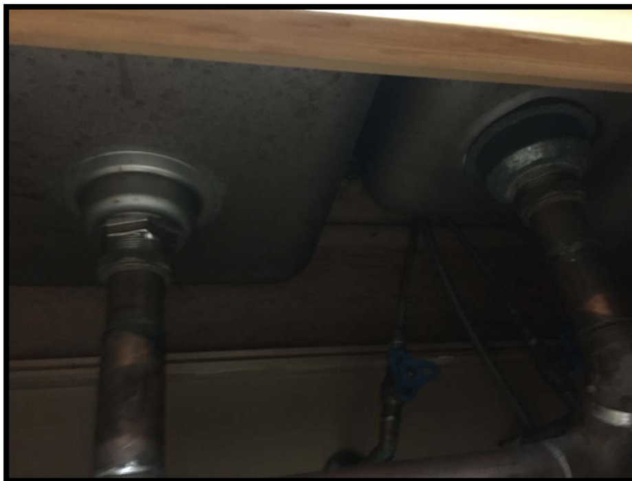
Photograph 2: Asbestos-Containing Silver Sink Undercoat.
