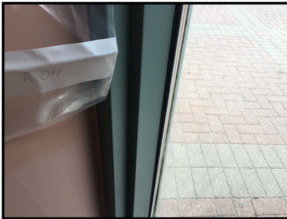
Photograph 2: Asbestos-Containing Black Window Caulking.
