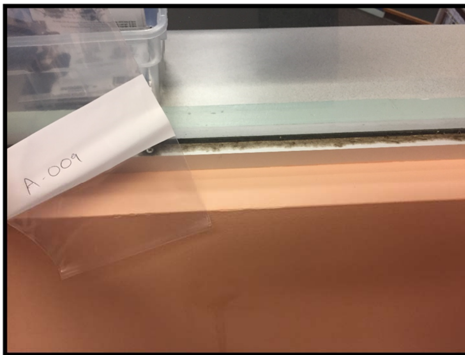
Photograph 1: Asbestos-Containing Black Window Caulking.
