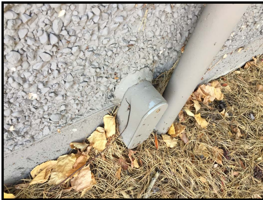
Photograph 1: Asbestos-Containing Brown Firestop.
