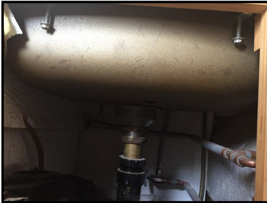
Photograph 1: Asbestos-Containing Gold Sink Undercoat.
