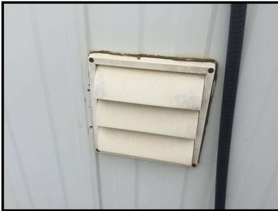
Photograph 2: Asbestos-Containing Brown Building Caulking.
