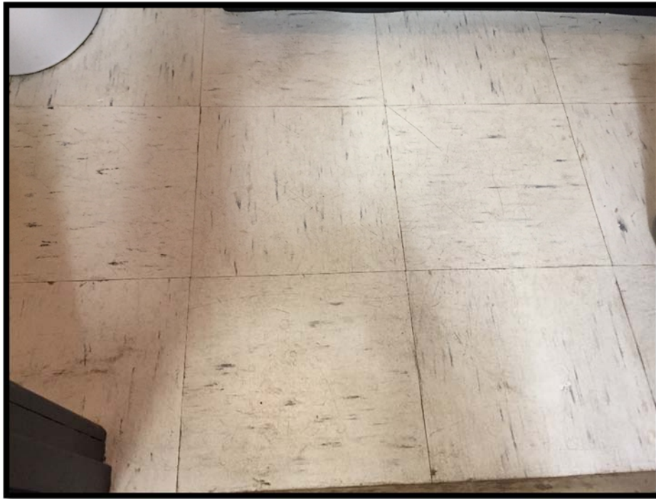
Photograph 1: Asbestos-Containing 1'x1' Off-White Floor Tile with Black Flecks.
