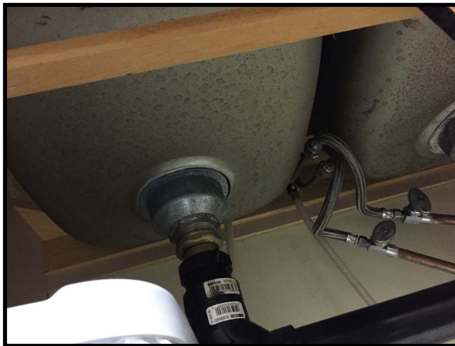
Photograph 2: Asbestos-Containing Silver Sink Undercoat.
