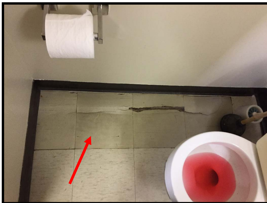
Photograph 1: Asbestos-Containing 12"x12" Beige Floor Tile with Black and White Streaks.
