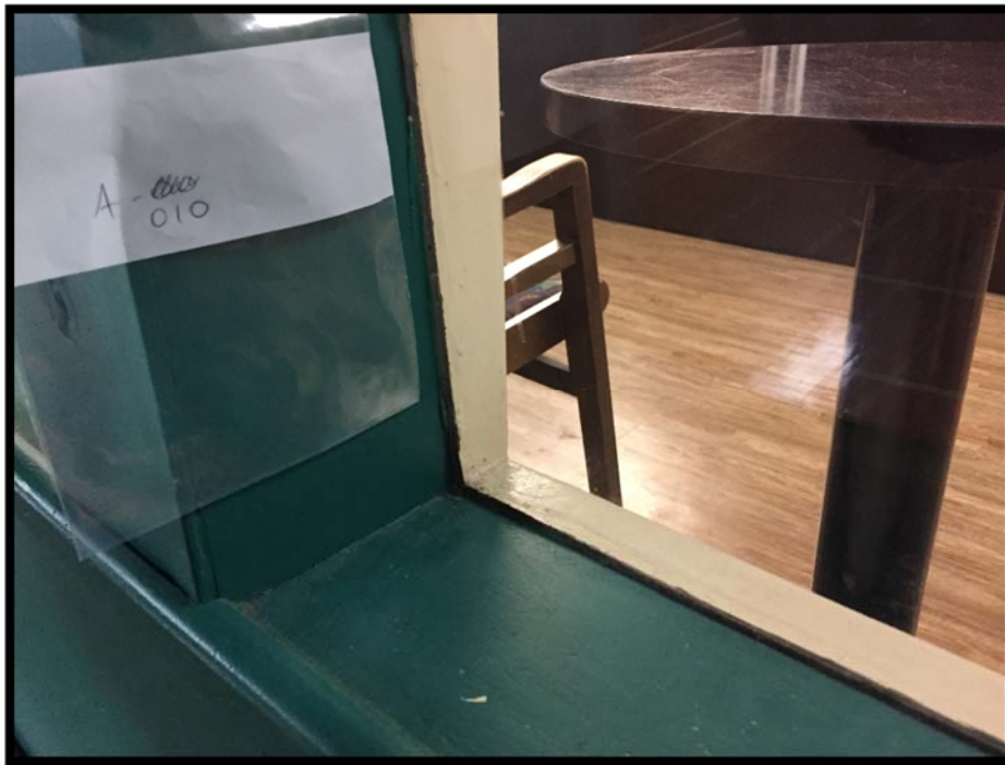
Photograph 2: Asbestos-Containing Black Window Caulking.
