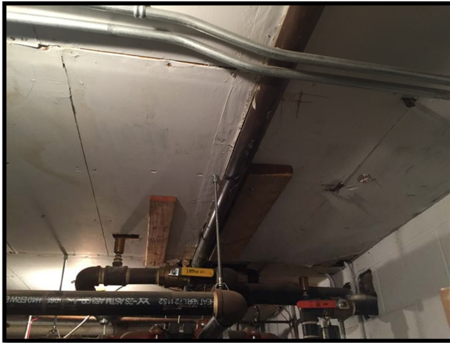
Photograph 1: Asbestos-Containing Drywall Joint Compound.
