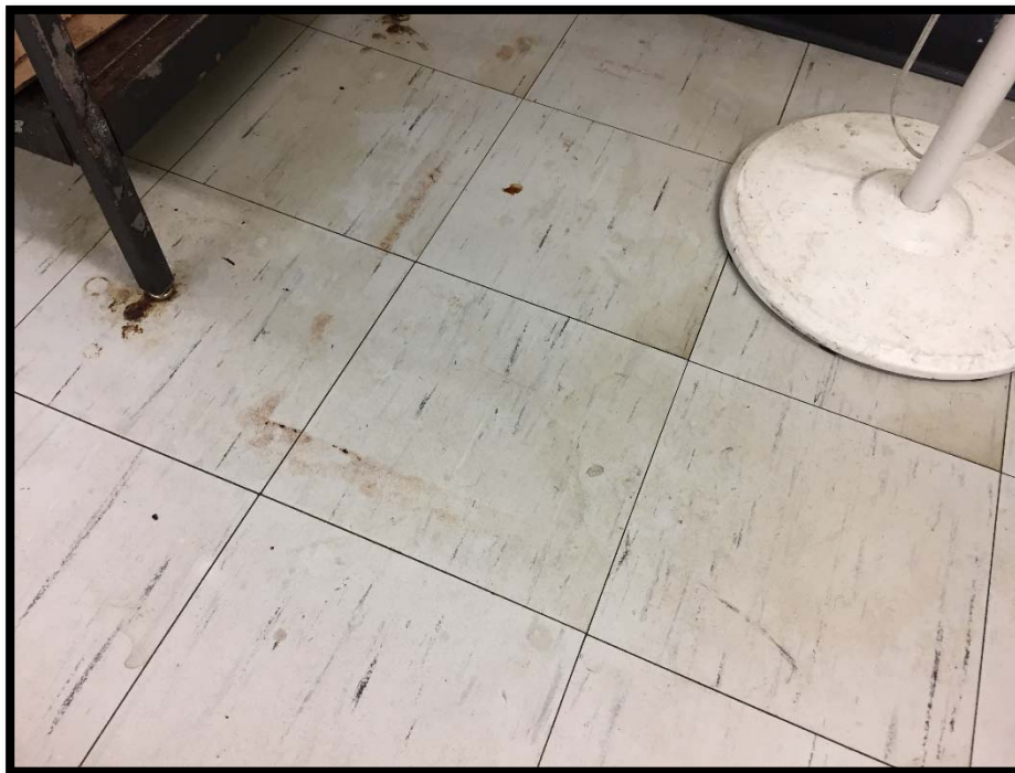
Photograph 1: Asbestos-Containing 12"x12" Off-White Floor Tile with Black Streaks.
