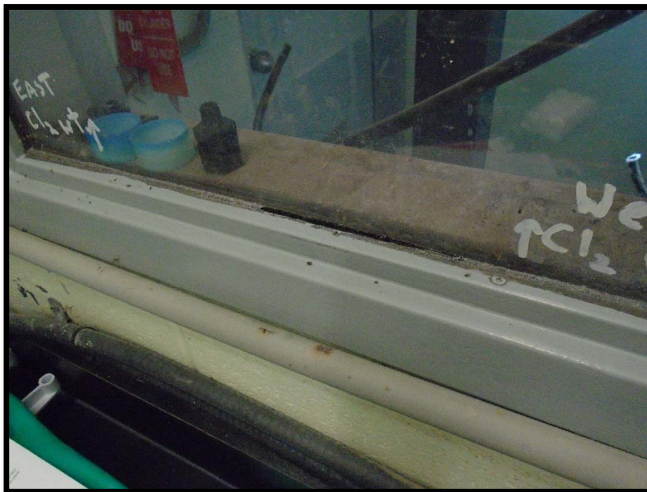
Photograph 4: Asbestos-Containing Black Window Putty.
