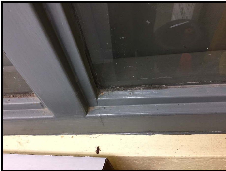
Photograph 3: Asbestos-Containing Grey Window Caulking.
