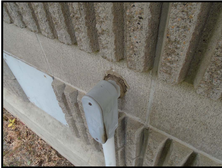
Photograph 6: Asbestos-Containing Light Grey Building Caulking.
