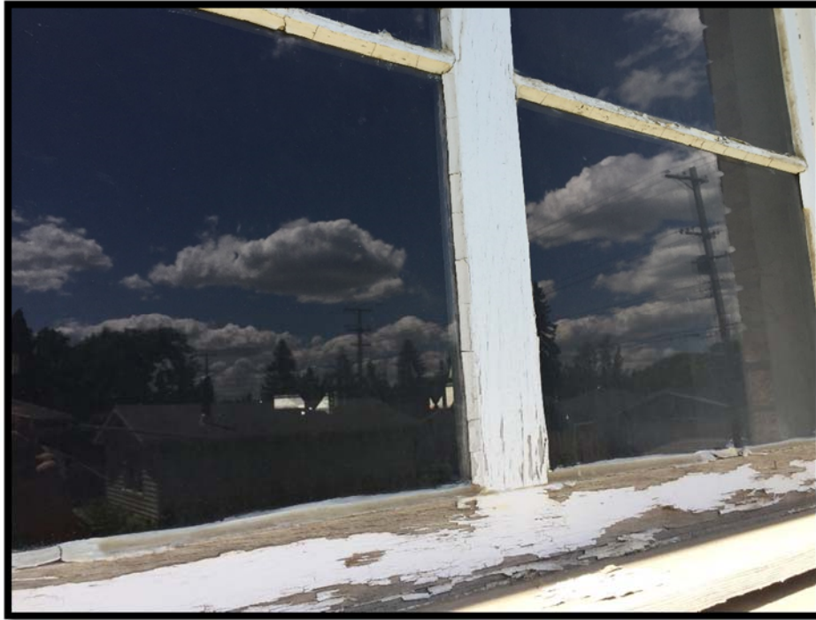
Photograph 1: Asbestos-Containing White Window Caulking.
