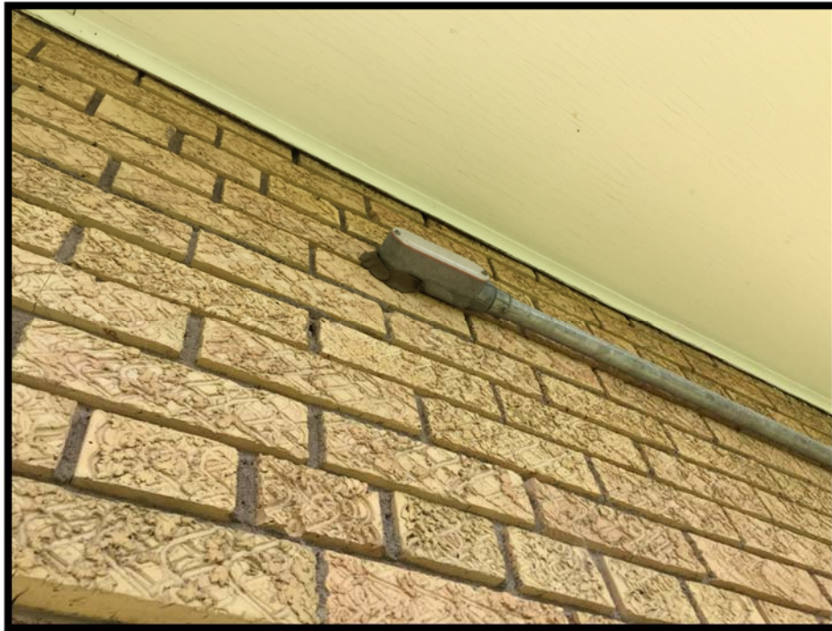
Photograph 2: Asbestos-Containing Black Firestop.
