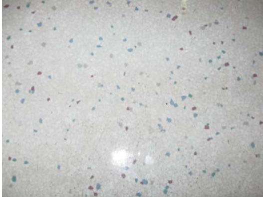
#1) Sheet Floor Covering
