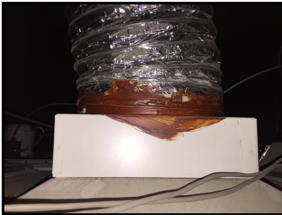
Photograph 2: Asbestos-Containing Red/Brown Duct Mastic.
