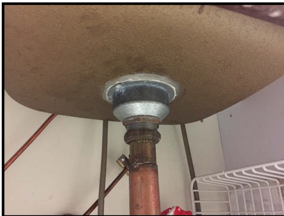
Photograph 1: Asbestos-Containing Gold/Silver Sink Undercoat.
