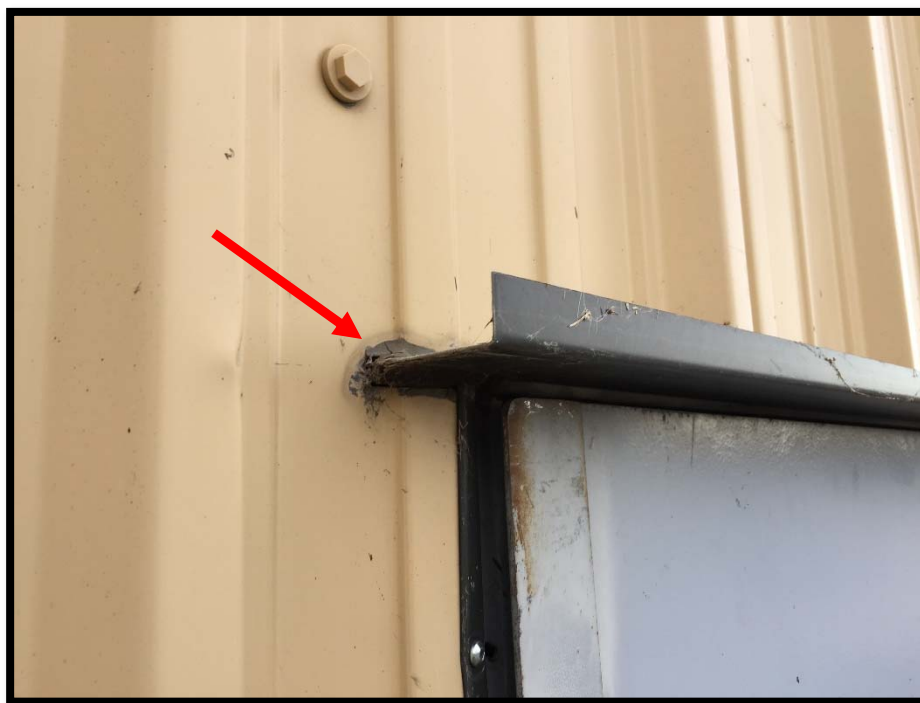
Photograph 1: Asbestos-Containing Black Door Caulking.
