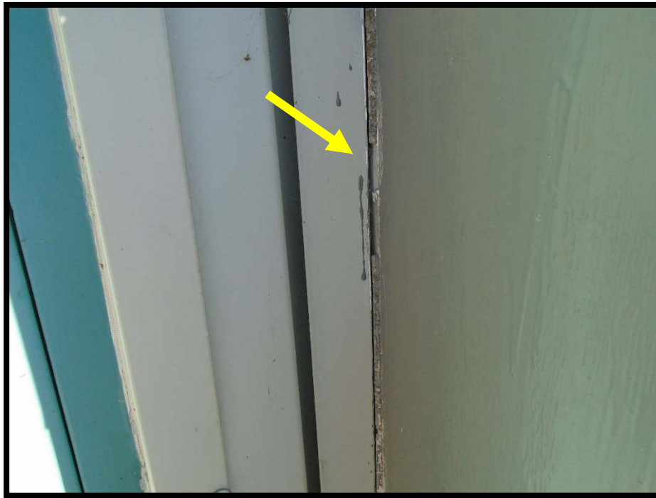
Photograph 1: Asbestos-Containing Grey Caulking
