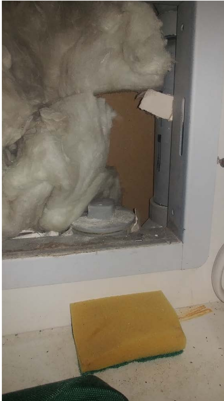
PHOTO 2 – Box Office Washroom- Wall Access Showing Fiberglass Insulation
