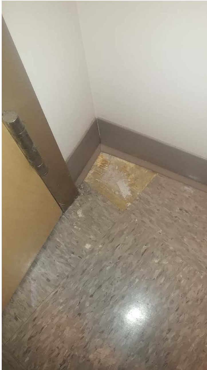
PHOTO 1 – Electrical Room Floor- Floor Tile Removed
