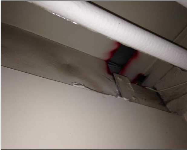
Photo 1 - Non-Asbestos containing fibreglass piping insulation on piping above acoustic ceiling tiles in hallway location 117.
