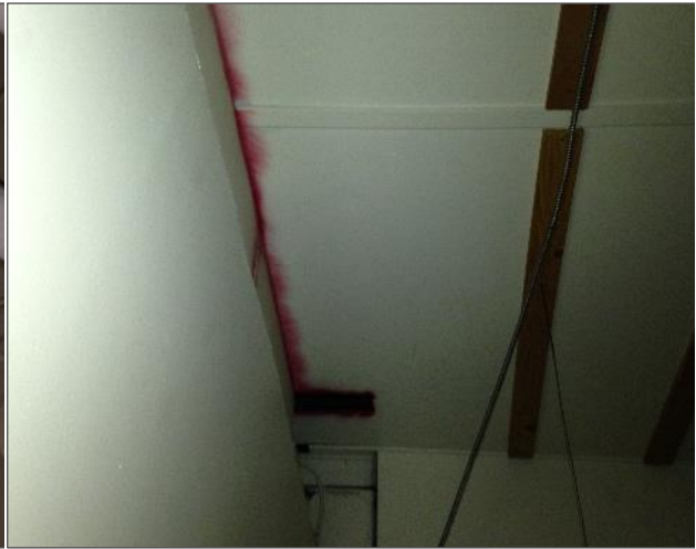
Photo 11 Asbestos-containing Transite panels across the ceiling.
