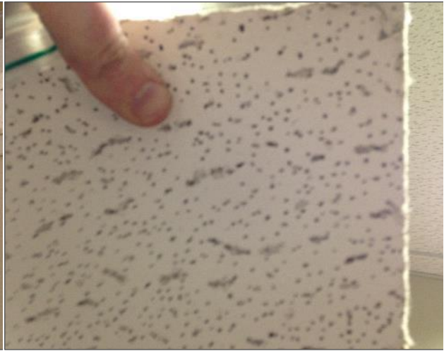
Photo 7: Acoustic Ceiling Tile, 24"x48" Pinhole and Fissure, Date Stamp 05/13/13, Office Location (119).
