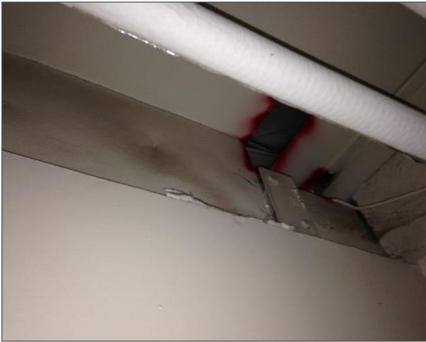
Photo 10 Asbestos-containing Transite panels above drywall along north exterior wall and across the ceiling. Non-asbestos containing fiberglass pipe insulation.
