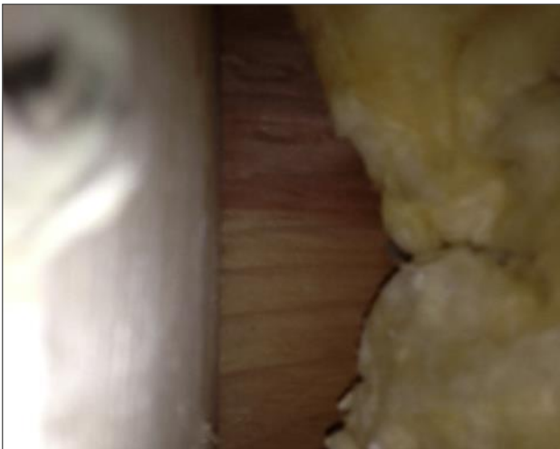
Photo 12 Intrusive hole through north exterior drywall wall (Below the transite board shown in Photo 10), fiberglass insulation, plywood exterior sheathed with metal siding.
