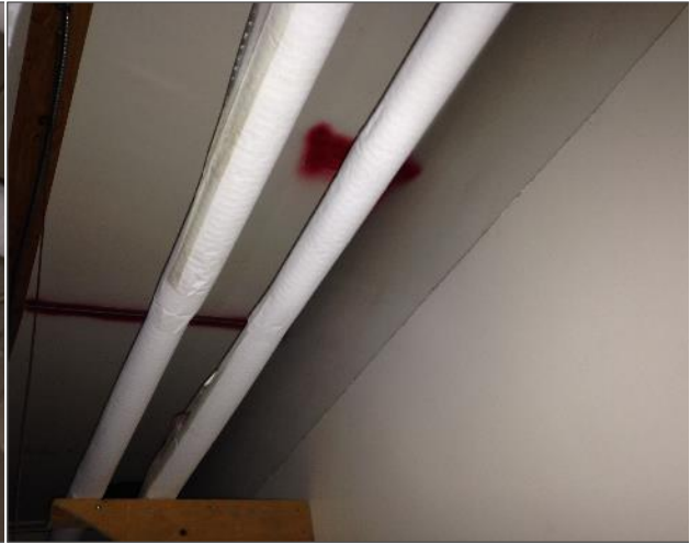
Photo 2 - Non-Asbestos containing fibreglass piping insulation on piping above acoustic ceiling tiles in hallway location 117.
