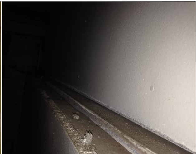
Photo 13 Asbestos-containing Transite panels along the top of the north exterior wall transition to drywall below.
