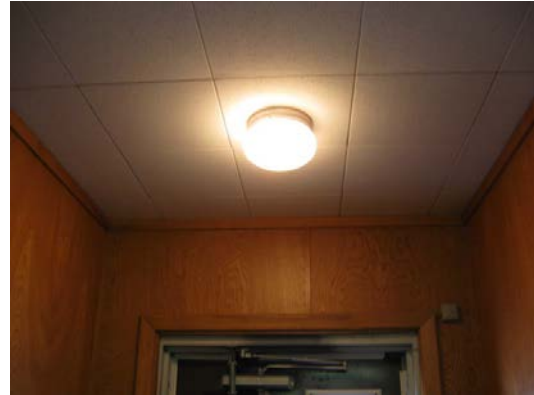
#7) Heat Shield in Light Fixture
