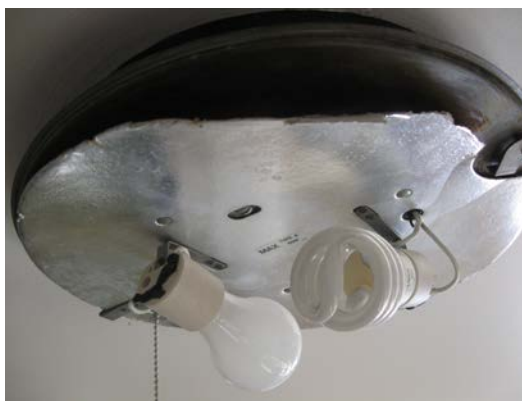
#7) Heat Shield in Light Fixture
