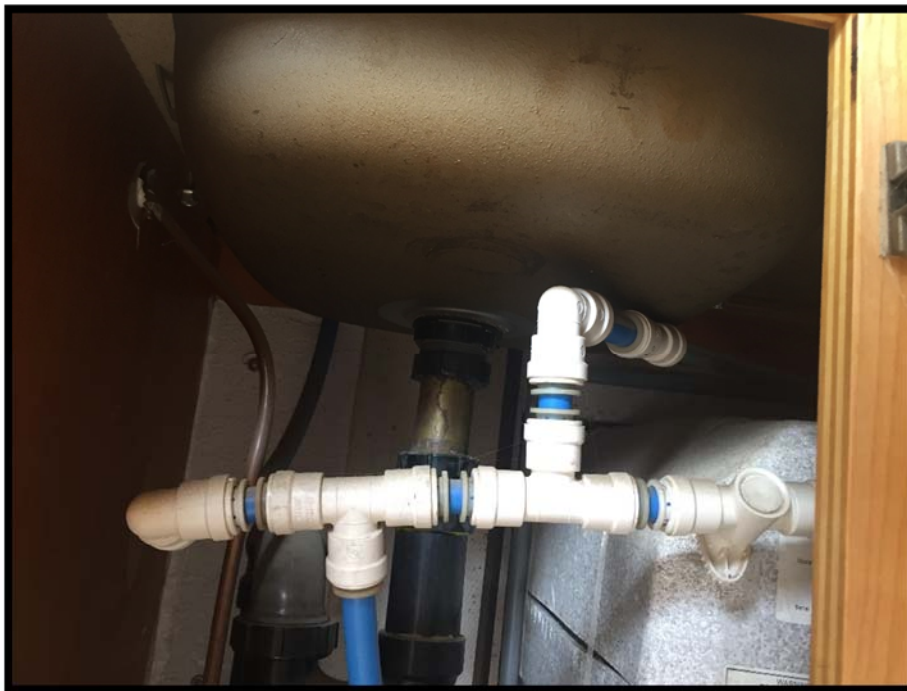
Photograph 1: Asbestos-Containing Gold Sink Undercoat.
