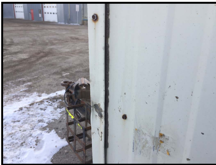
Photograph 3: Asbestos-Containing Black Building Caulking.
