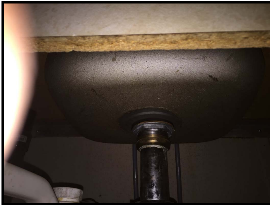
Photograph 2: Asbestos-Containing Silver Sink Undercoat.
