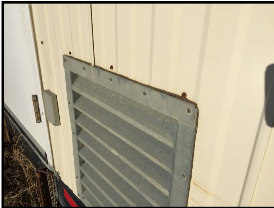
Photograph 2: Asbestos-containing Black Building Caulking.
