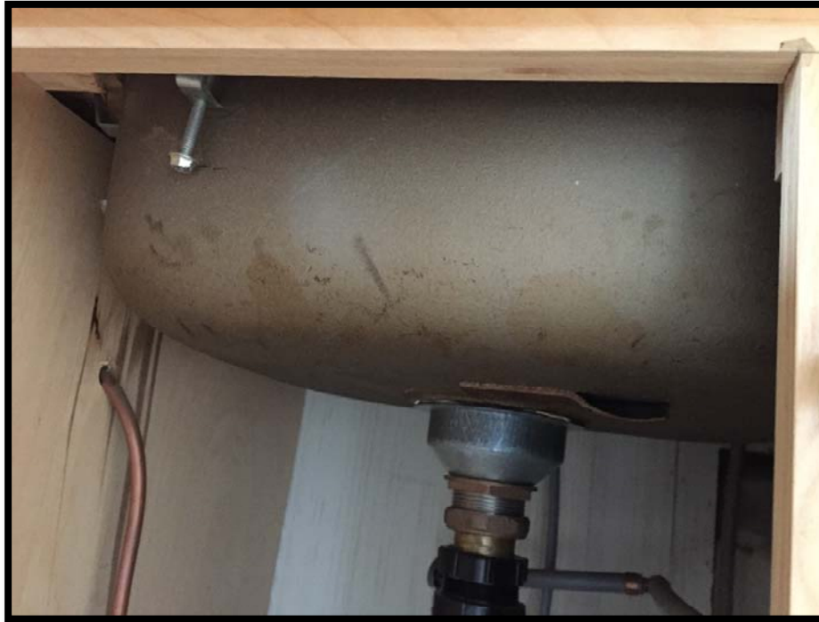
Photograph 1: Asbestos-Containing Gold Sink Undercoat.
