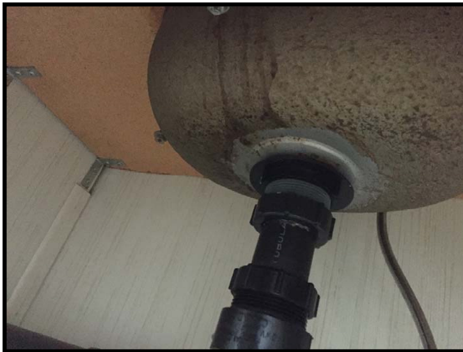
Photograph 1: Asbestos-Containing Silver Sink Undercoat.
