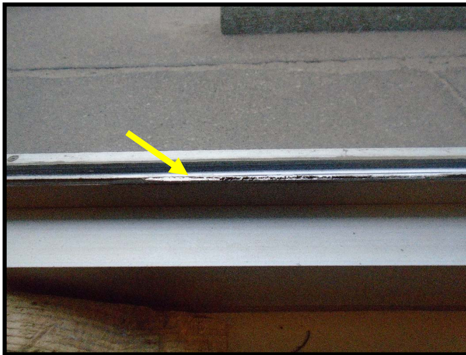
Photograph 1: Asbestos-Containing Black Window Caulking.
