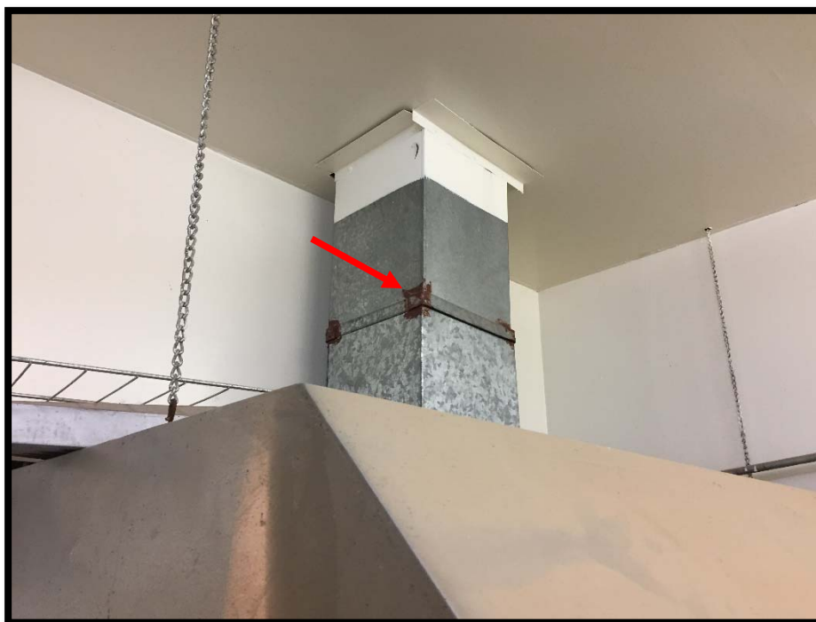
Photograph 1: Asbestos-Containing Red/Brown Duct Mastic.
